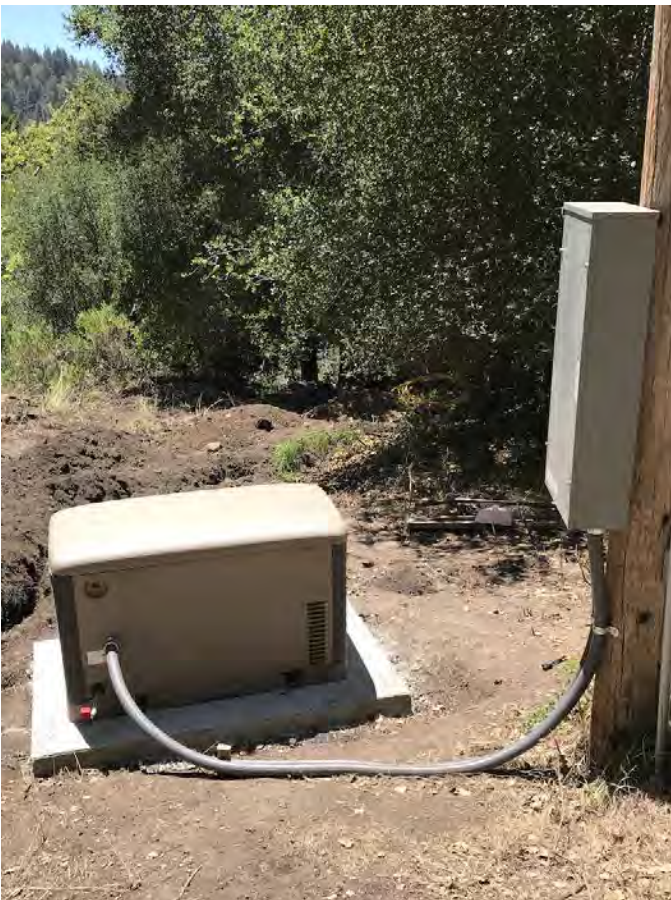
New generator for Drubdra (3-Year Retreat Center)
